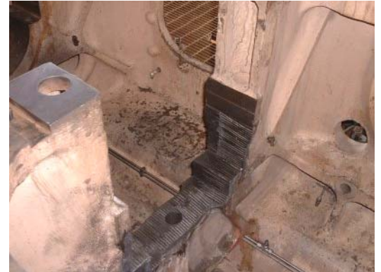
Main Bearing Pocket Section Removed
